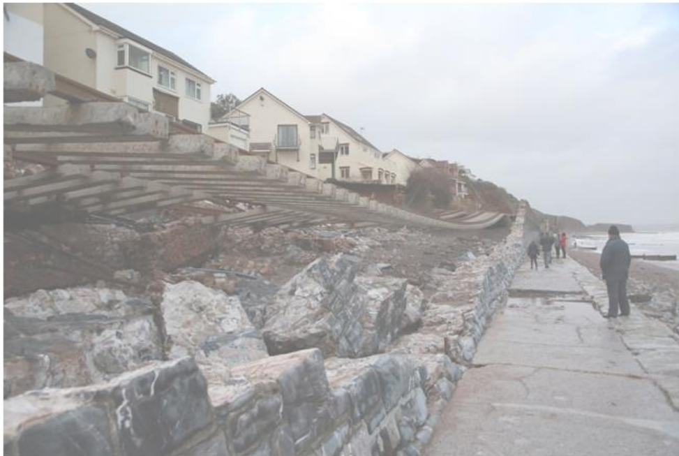
This image shows the south-west main-line railway at Dawlish, Devon, suspended in mid-air after the foundations were washed away by the storm of 5 February. Photograph courtesy Matt Clark, Met Office
